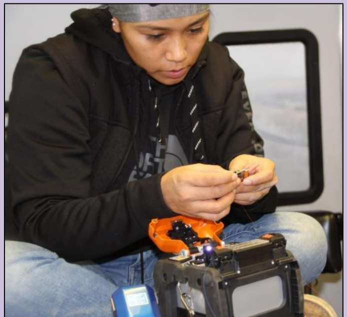
Joey Casady and Kayonnie Badonie cut and splice our fiber optic cables from our damaged building to our temporary offices allowing us to be back online within hours.
